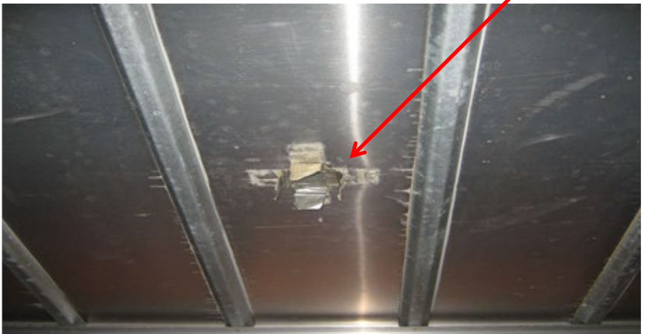
Improper roof repair
